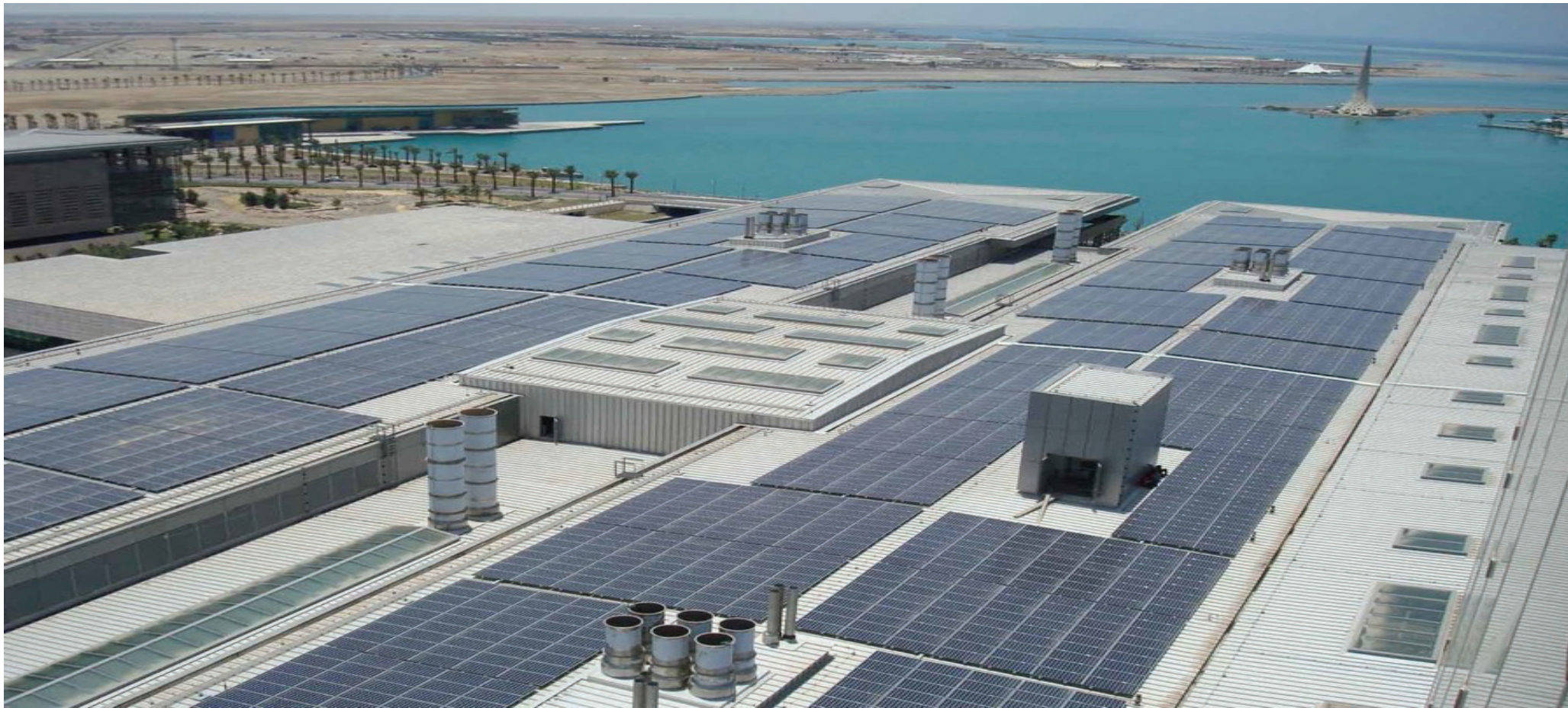
2-MW Roof-top Solar PV plant at KAUST
